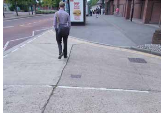
Poor quality surface materials
